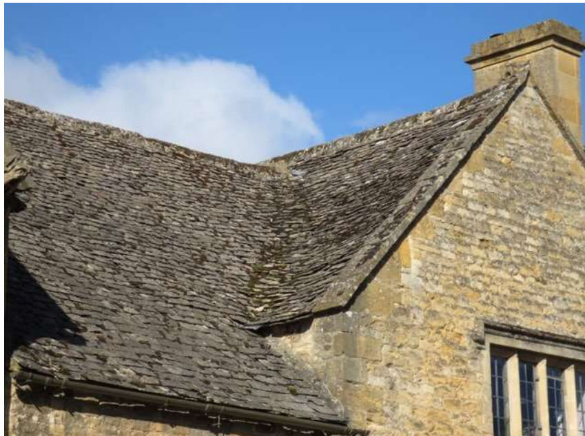
Fig.1. A traditional Cotswold stone roof showing the stone-tiles diminishing in size towards the ridge and a ‘swept valley’ at the junction with the dormer.
